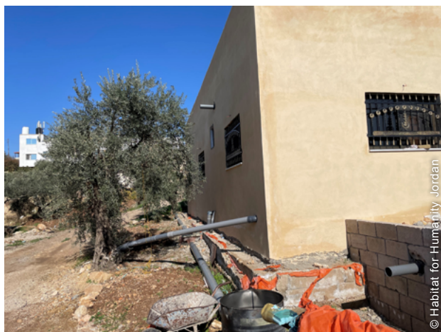
Among the upgrades, greywater reuse systems were installed, for instance to irrigate trees and gardens and reduce the pressure on local water systems.
