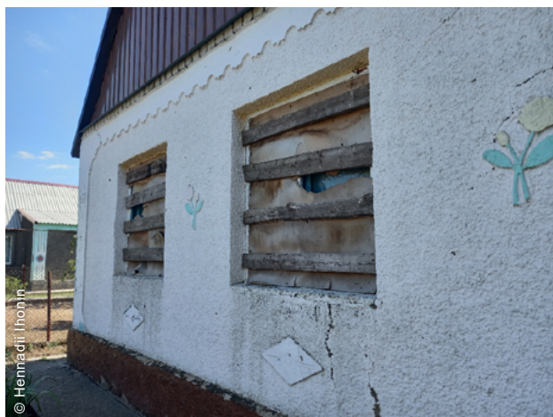
Dwellings with light and medium damage were selected. Typical damage included windows and doors, roofing, and exterior walls.
