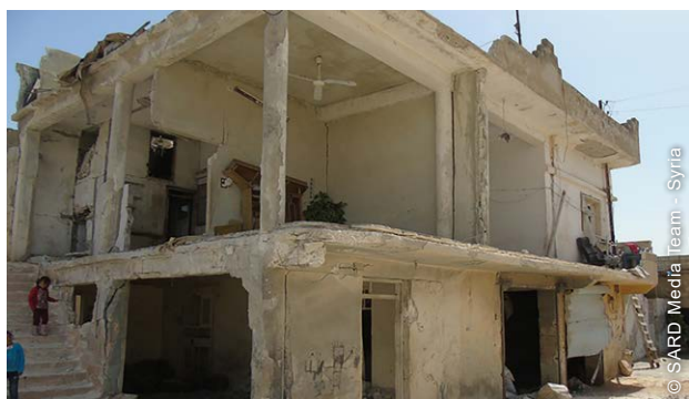
Many IDP, returnee and vulnerable local households were living in significantly damaged homes.
