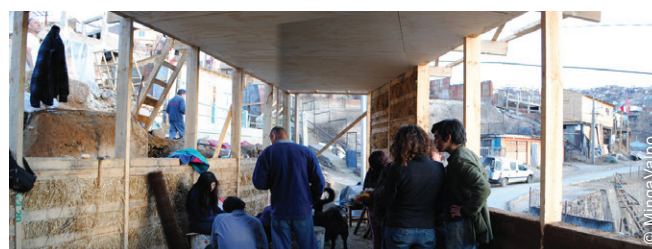
Local groups of architects organized building workshops to rebuild some of the houses affected by the fire on the Quebradas.
